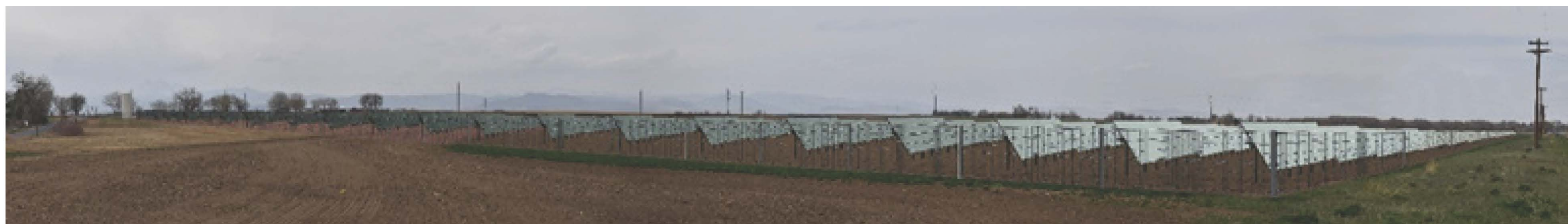
4- Solar Arrays Looking Northwest from C.R. 34 & C.R. 5.
